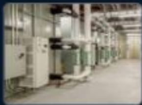
Building management systems
